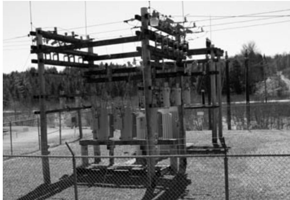
If approved by the voters, WEC's substation near Maple Corner will be replaced by a more modern, energy-efficient facility with environmental protections for nearby wet areas.
