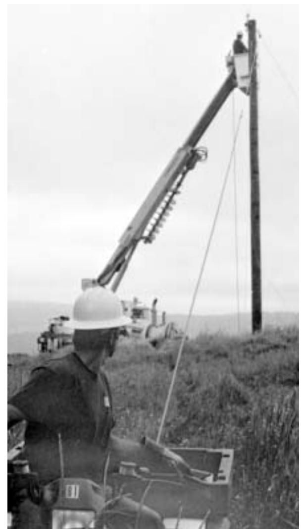
Tim Pudvah, foreground, pulls the end of a new section of power line with a six-wheeler. As Tim drove forward, the slack line along a series of poles rose into place.
