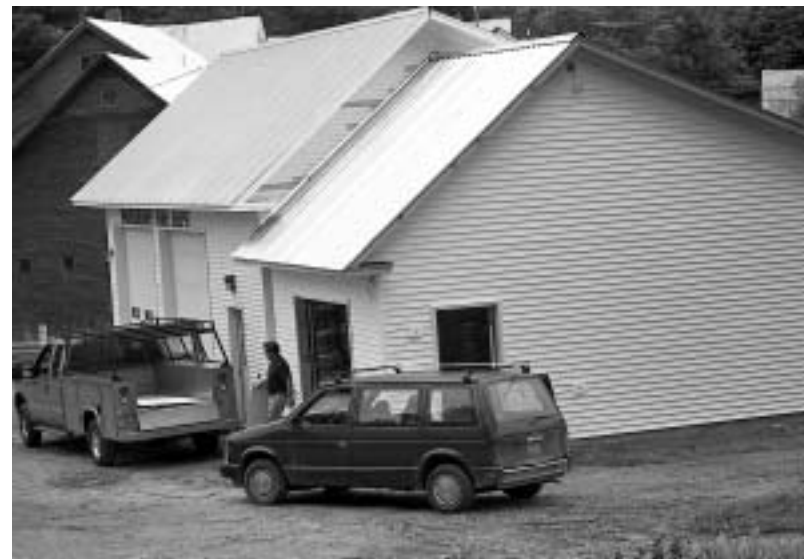
Volunteer Peter Peltz unloads construction materials at the new site for the Woodbury/Calais Foodshelf. WEC donated $500 for the project from its Community Fund.
