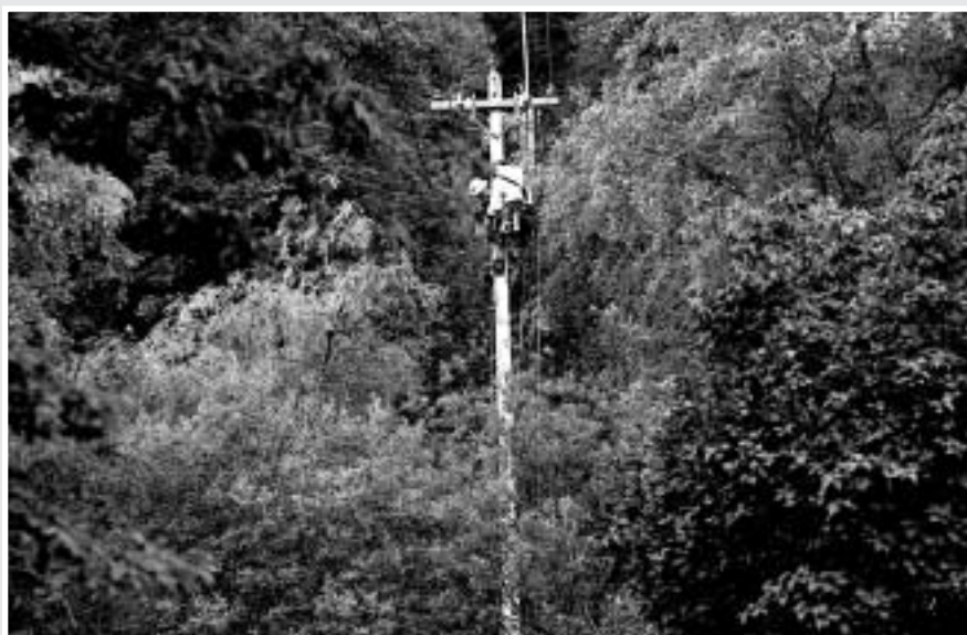
Rich Hallstrom and Mark Maloney, working to improve power quality in East Roxbury.
