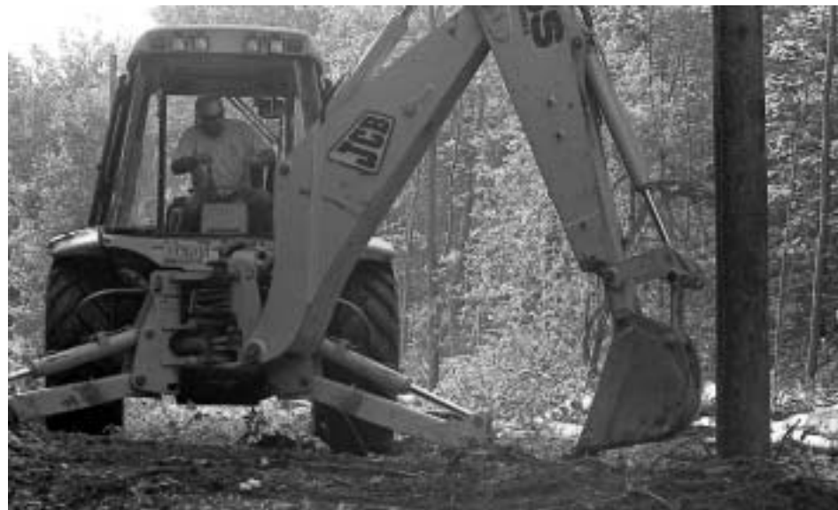
Foreman Bob Fair at the controls of a backhoe, tidying up new right-of-way in Washington. Co-op linemen master a variety of skills in their work.
