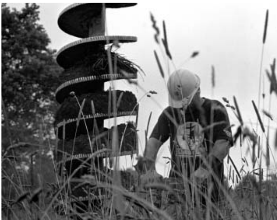
Ray Hall, at work on a hole for a new utility pole in Williamstown.
