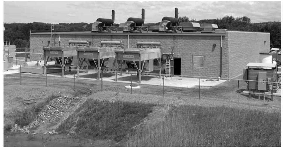
The generating station at the Coventry landfill, now in operation.
