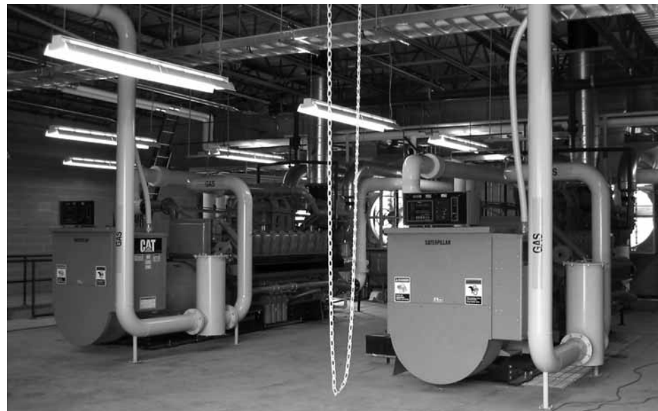
Caterpillar engines in WEC's power house at the Coventry landfill. Once fine-tuning is completed, the engines, which are fueled by methane captured from the landfill, will produce 4.8 megawatts of power for WEC members.
