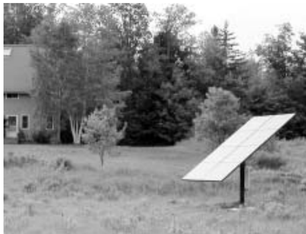
A small solar array in the yard can produce half of this homeowner's power.
