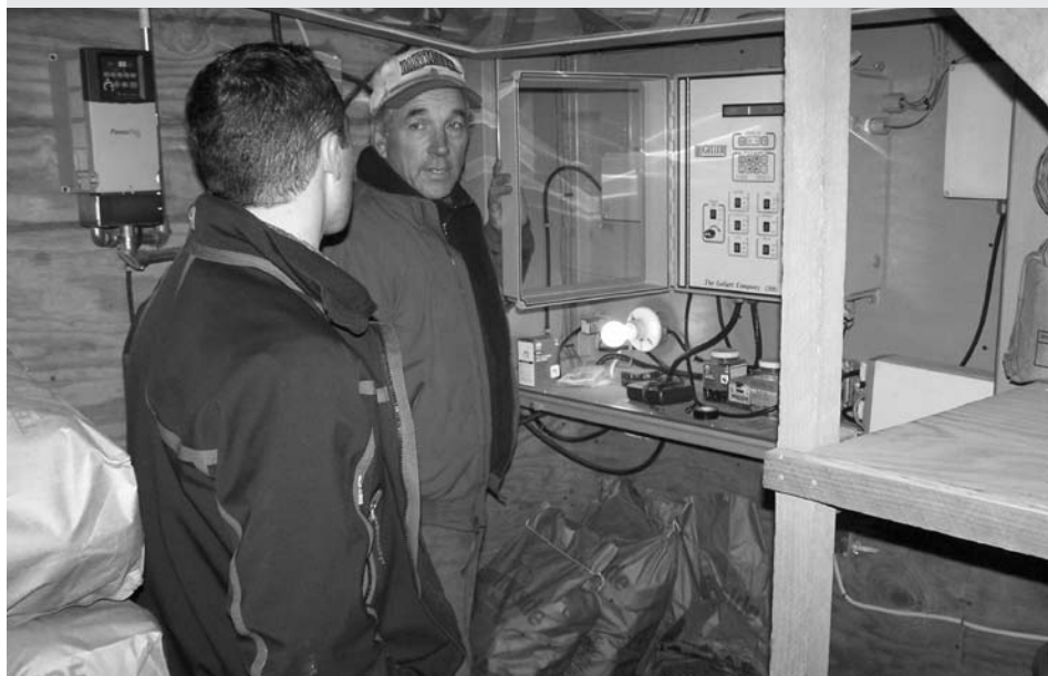
Above, Williamstown potato farmer Bob Chappelle (in cap) describes his packaging machinery to Taurin Spaulding of Efficiency Vermont. With assistance from EVT and Washington Electric, Chappelle installed equipment that reduces his energy usage and improves his storage operation. Below, Chappelle and Spaulding at the new control panel. (photos by Bill Powell)
