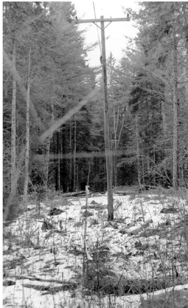
Many power line corridors that were built across the countryside decades ago are now hard for linemen to reach and repair in outages – a situation the Co-op is working to improve.
