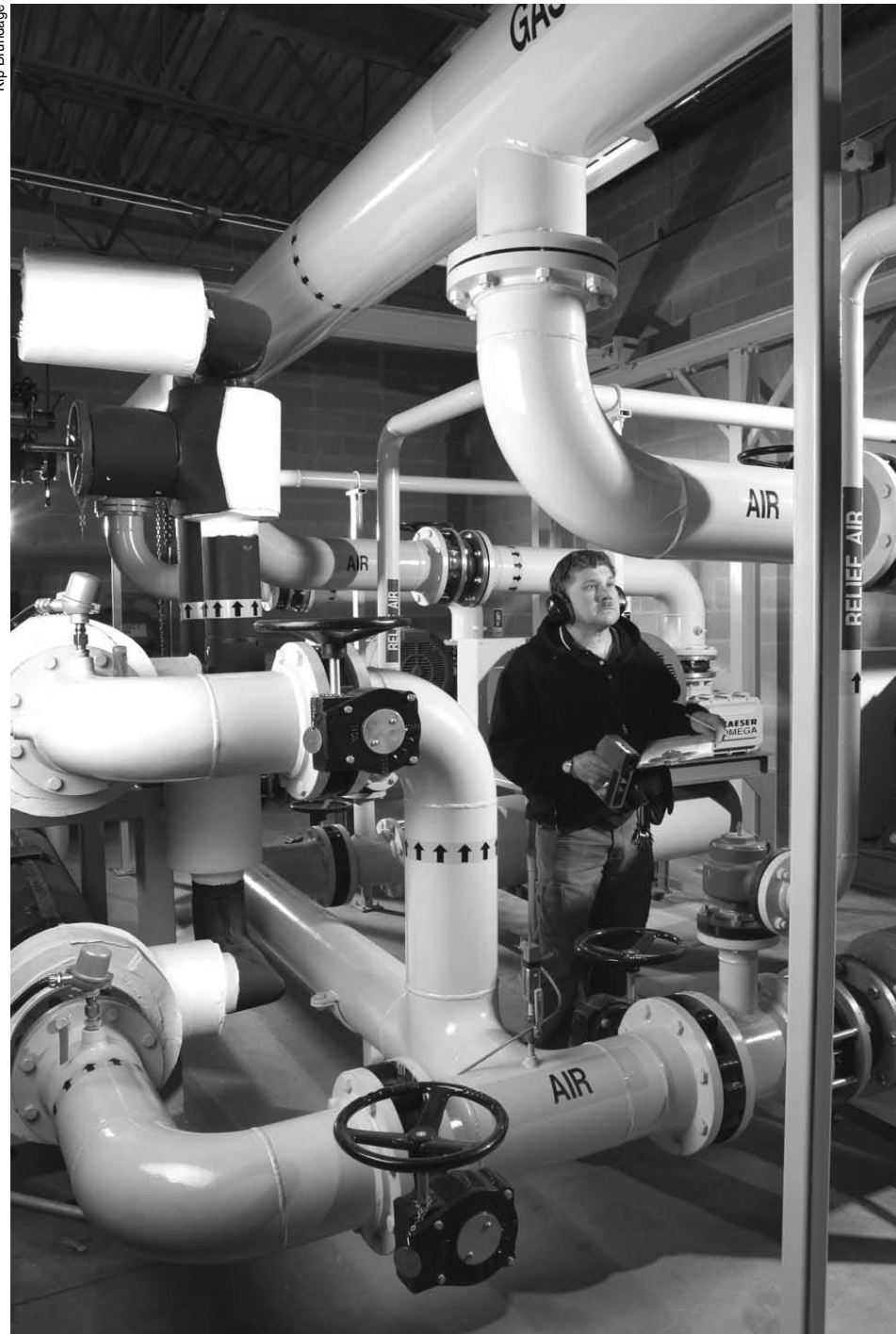
Plant Operator Scott Wilson has been fine-tuning WEC's electric-generation facility in Coventry. Under Scott's watchful eye, the plant has become increasingly productive.
