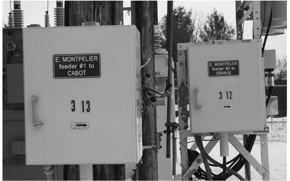
Reclosers at the East Montpelier substation. One monitors the three-phase "feeder" line to Cabot, the other monitors the feeder to Orange. These reclosers help avoid outages, and can also tell a repair crew how far out from the substation a "fault" has occurred.
