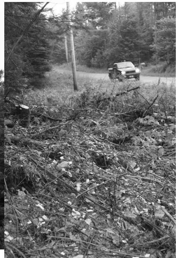
The very definition of a "danger tree" (left), this weakened, dying fir leans over the power line on Pike Hill Road in Corinth. It's on the Co-op's list for removal. In the woods, cleared brush is stacked along the right-of-way, but where the lines run beside the road, as on Miller Road (Corinth, below) the trunks and branches are chipped and cleared away.
