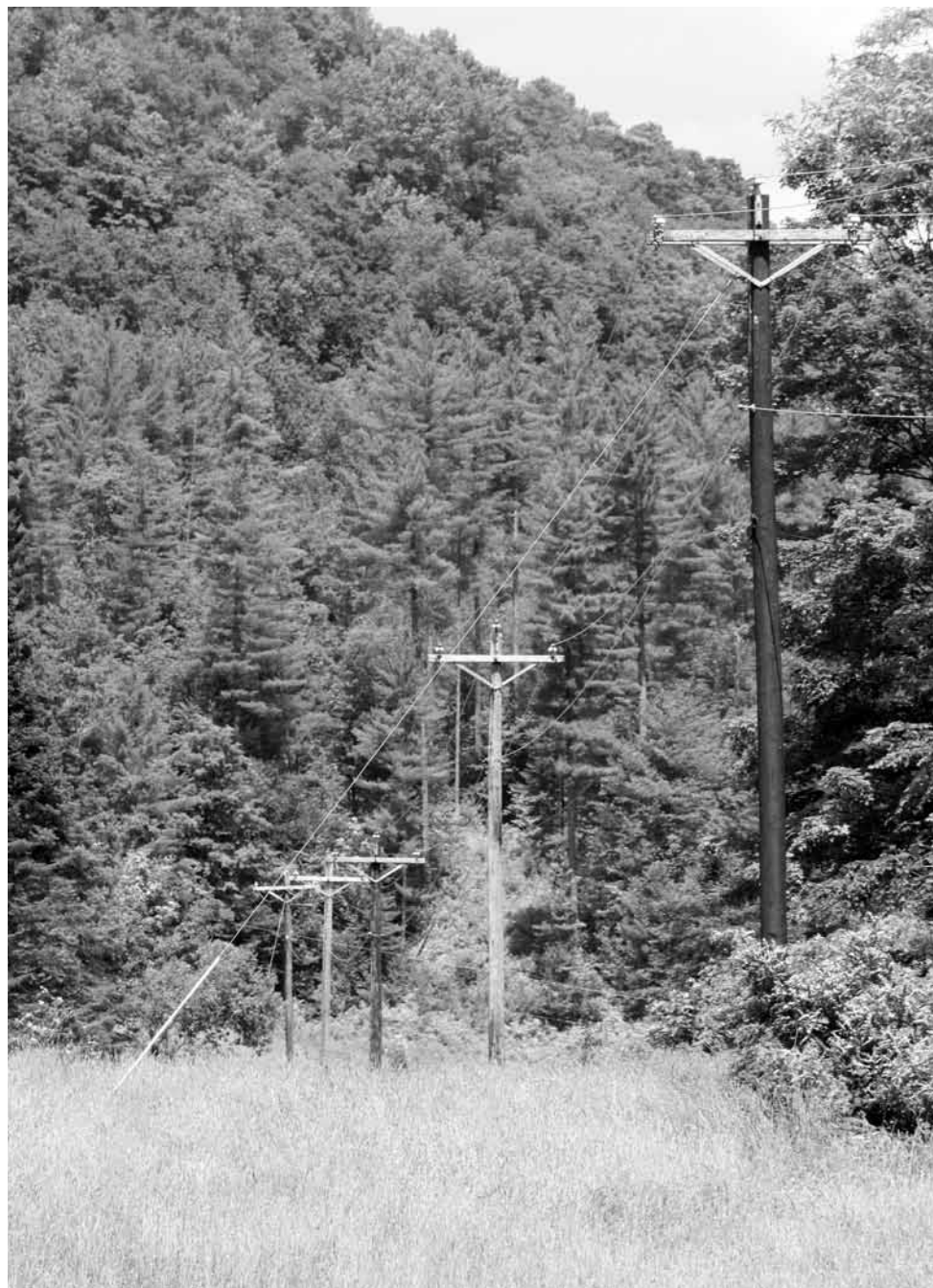
A section of three-phase power line, recently reconstructed by WEC with spanking new poles and wires, comes marching over the hills in Chelsea.
