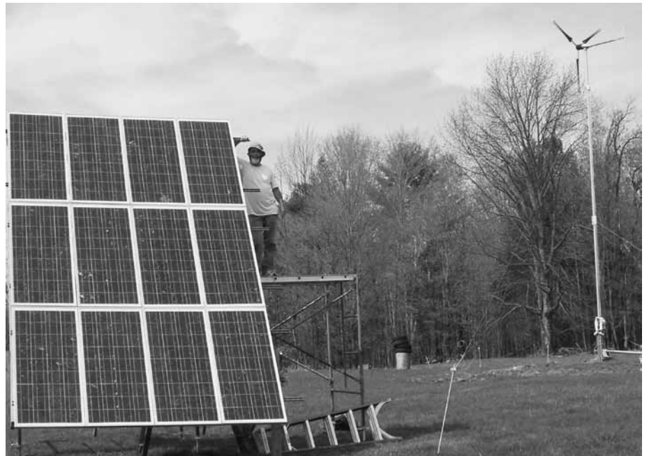
WEC member Ed Hutchinson stands proudly on a construction scaffold behind his 1.3- kW solar array. The power generated by this 12-panel array and the 1-kW wind turbine on the right goes to a battery bank in Ed and Alexandra Thayer's basement.
