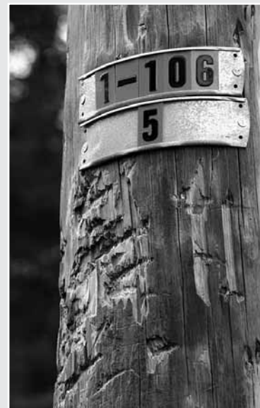
Ursine tooth marks on a WEC power pole.
