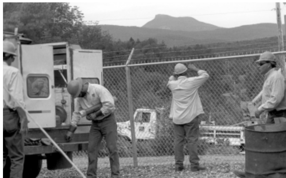
A busy morning, as WEC operations personnel prepare the Co-op's new Moretown substation for its July 10 start-up. Camel's Hump provides the scenery.
