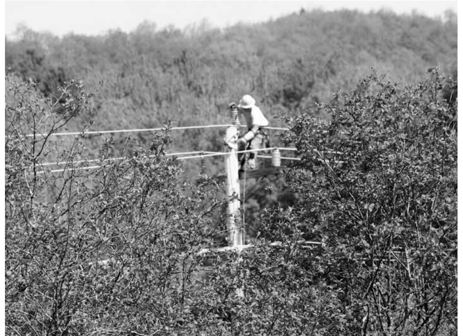
Line Foreman Tim Pudvah at work in the forest canopy off the County Road in East Montpelier. The veteran WEC lineman is shown replacing transmission-line insulators, part of a project to replace 495 of them this summer.
