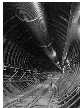
Workers construct the tunnel and rail system penetrating Yucca Mountain in Nevada.
