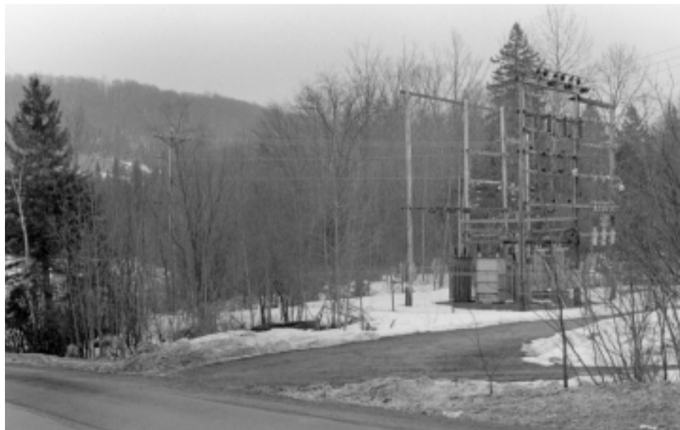
WEC's South Walden substation on the Cabot Road would soon be replaced by an up-to-date facility, with the approval of the voters at the Co-op's annual meeting.
