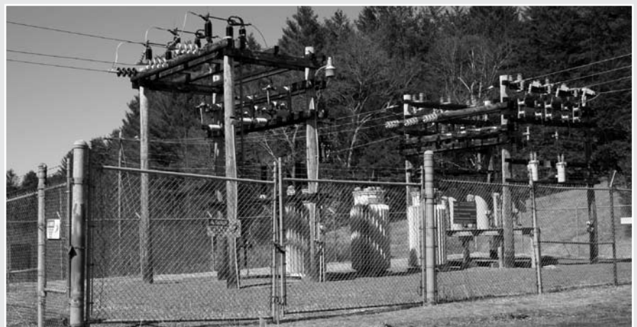
If approved by the voters, WEC's substation near Maple Corner will be replaced by a more modern, energy-efficient facility with environmental protections for nearby wet areas. The substation replacement project will be on your 2006 Co-op ballot.
