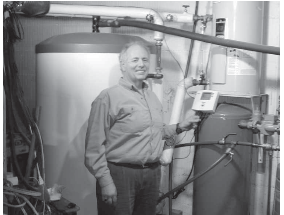
Bob Atchinson, with the tanks and apparatus that control his solar hot water system in Plainfield.
