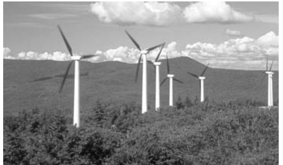
Green Mountain Power Corp.'s wind farm in Searsburg is Vermont's first wind-electric installation.
