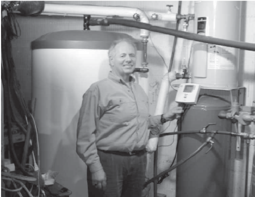
Bob Atchinson, with the tanks and apparatus that control his solar hot water system in Plainfield.
